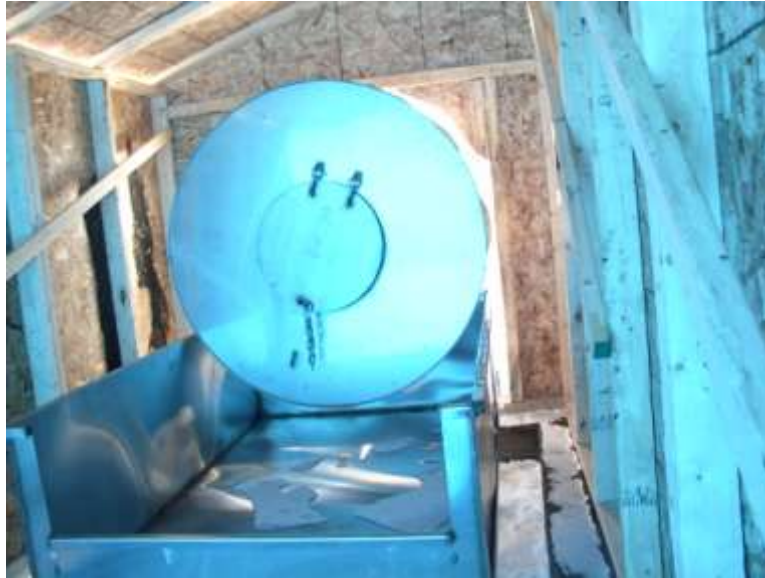
Photo 2: Biovator™ effluent opening and collector basin
